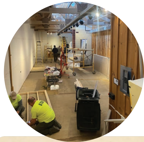
Fabrication In Full Swing The Forest Preserves construction department installing drywall and building partitions.
