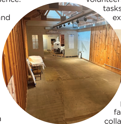
The Guttled Gallery Space Demolition is nearly completed, and fabrication is about to begin.
